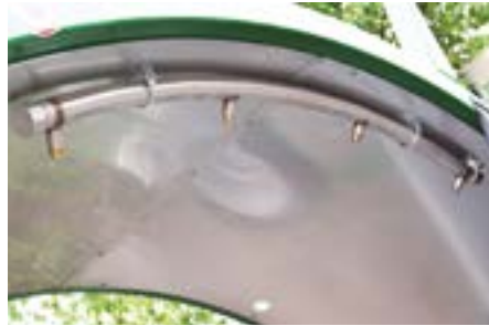
Water sprayer with nozzles. To achieve an optimal microorganism climate within the mound, the addition of water is essential.
